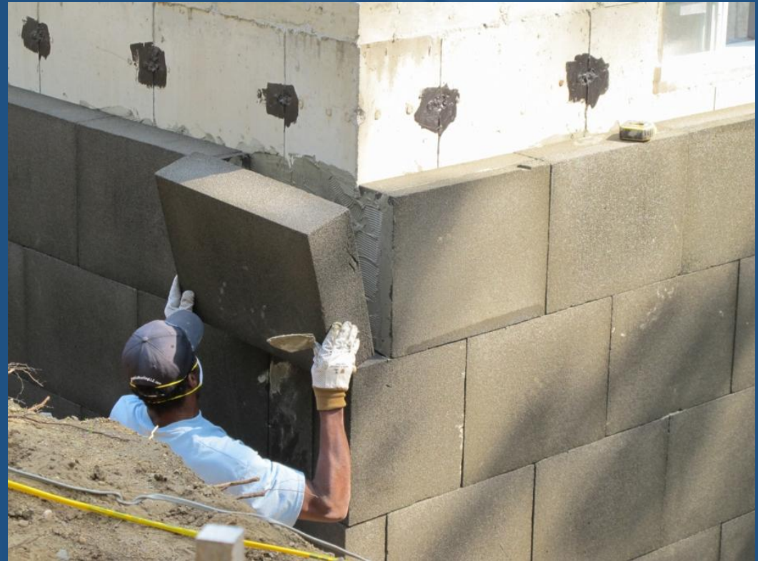
6" layer adhered onto foundation walls (R-21) with an Ardex X-5 polymer cement Photos: Alex Wilson
