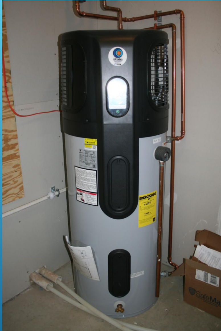
HEAT PUMP HOT WATER HEATER
