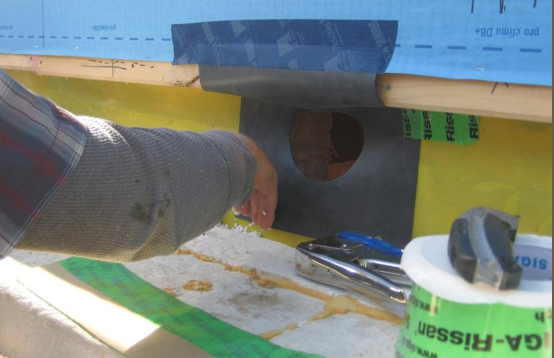
CERV Supply and Exhaust Penetrations
