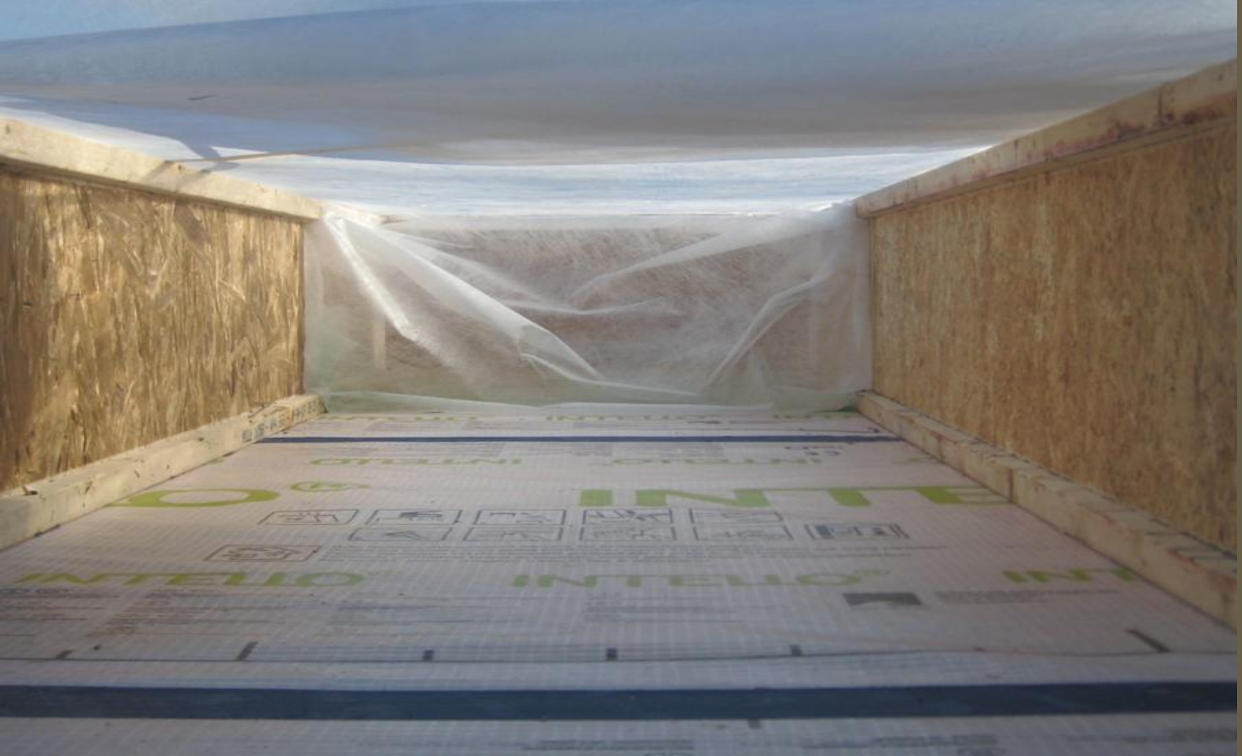
DP Cellulose Thermal Envelope Sensors and Moisture Meter Extensions 3 ft x 16" roof cavity
