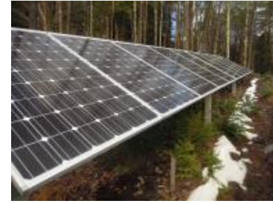
Solar PV System
