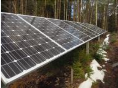
Solar PV System
