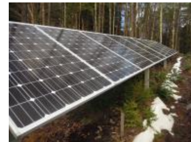
Solar PV System
