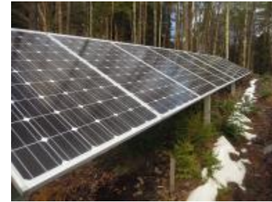
Solar PV System
