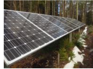
Solar PV System
