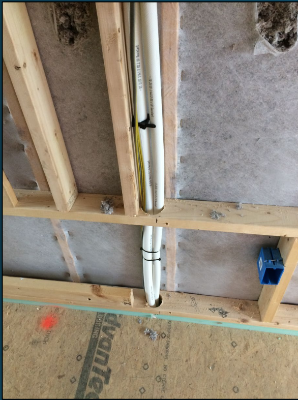
Heat pump tubing
