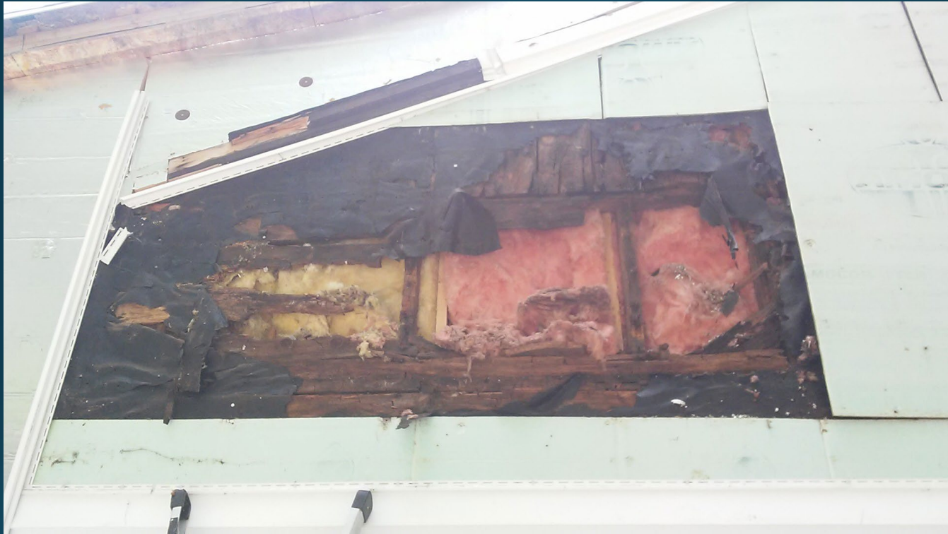
Insufficient exterior XPS sheathing, dirt floor basement
