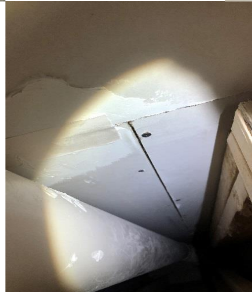
Pipe chase with seam missing tape
