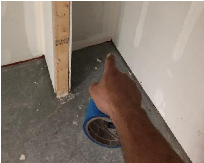
Drywall is not continuous behind interior partitions, resulting in leaks.
