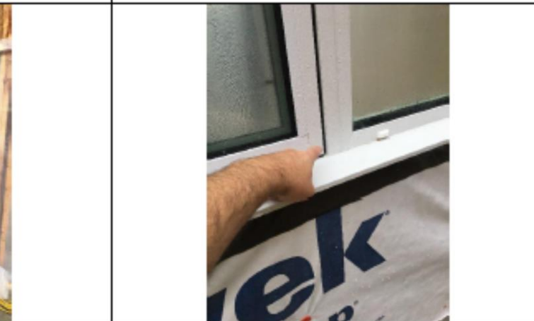
Fog wisped out at the lower corner of the sash even though the cam lock was engaged. This is not a major concern but highlights the importance of making sure the frames are installed square so the sashes close as they were designed to.
