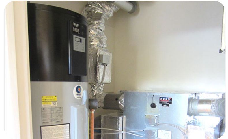
Heat pump water heater
