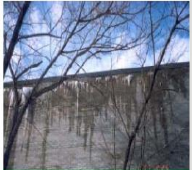
Figure 2: Ice forming on exterior of building.
