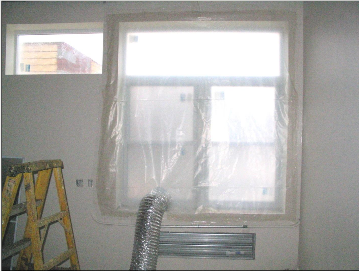
Window gaskets and AHUs both failed
