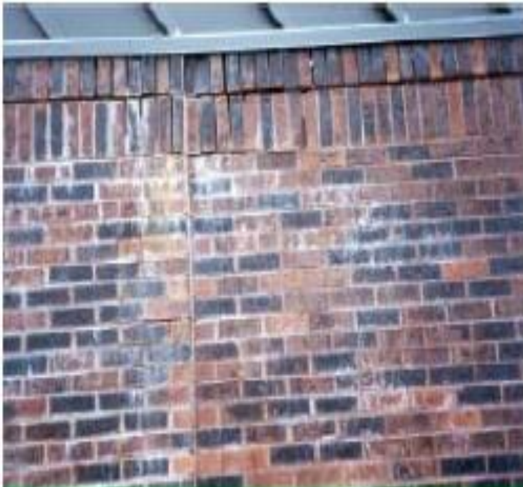
Figure 1: Efflorescence and spalling of bricks and mortar.
